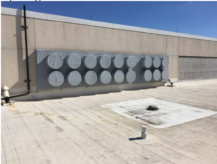
Taps for bypass unit
