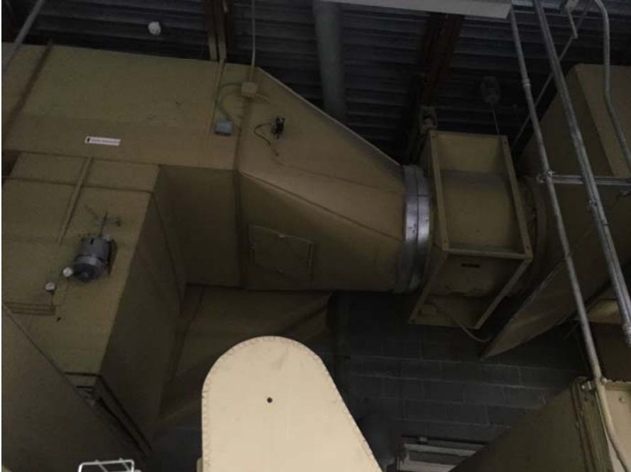
Pictures of AHU room P107:
