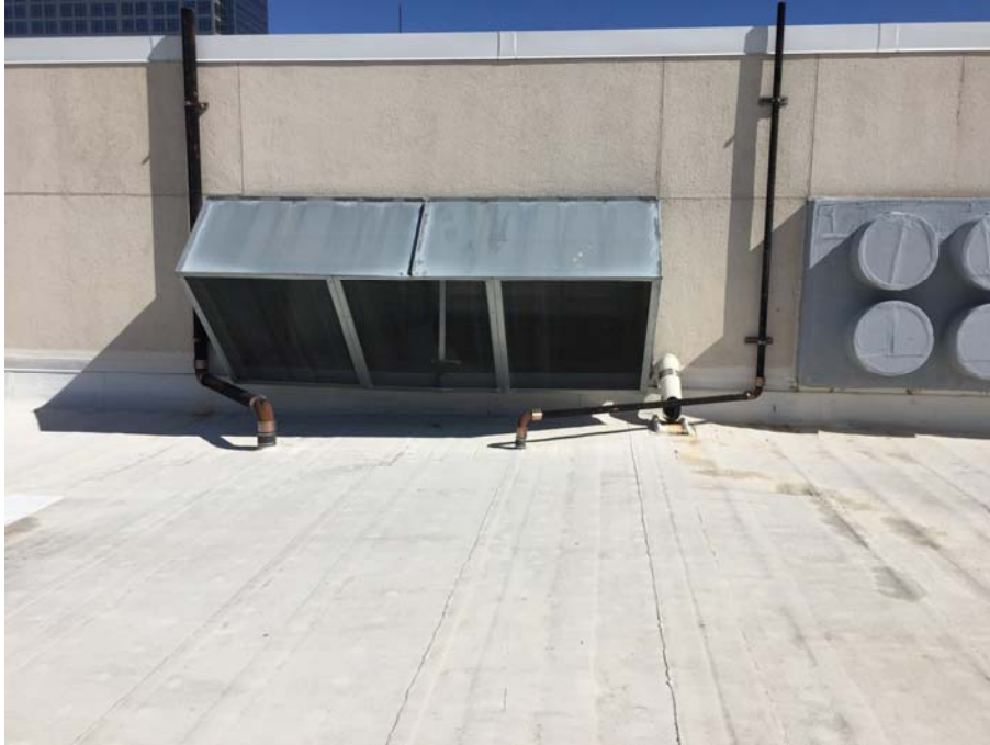
Outside air for bypass unit:
