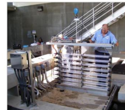
UV lamps in water treatment
